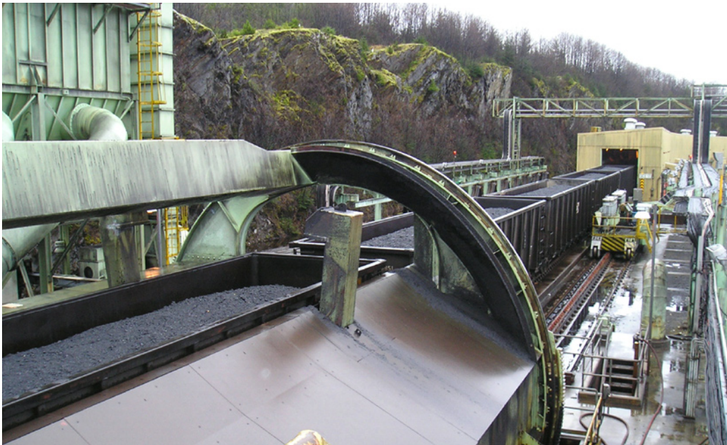
Continuous rotary rail car dumper and coal transfer at Prince Rupert
